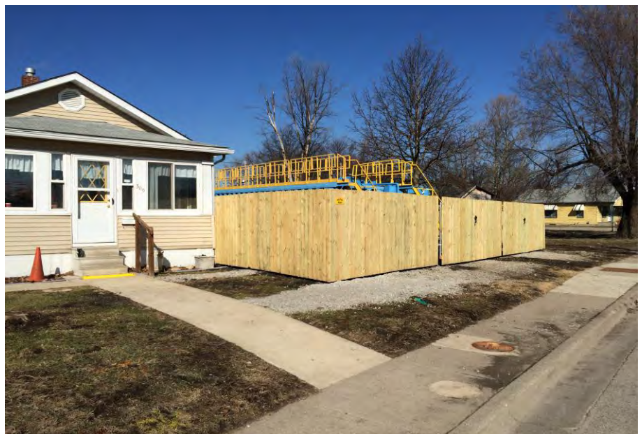
A privacy fence was installed around cleanup equipment to comply with a village ordinance.
