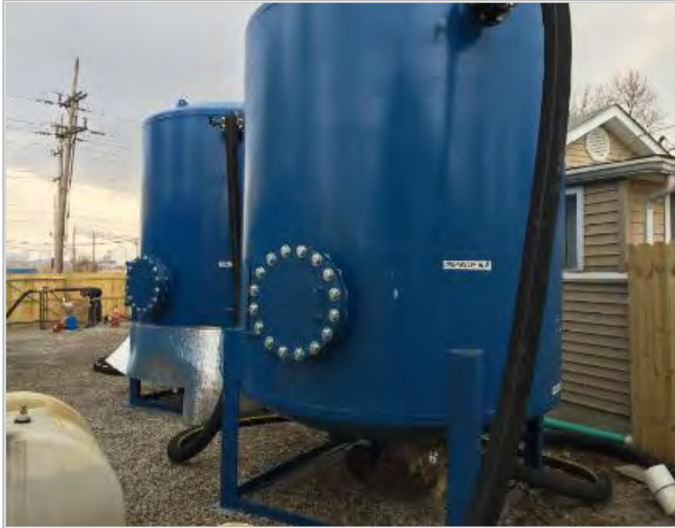
Activated carbon vessels used for the focused groundwater pumping pilot test.
