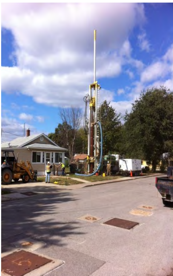
Some wells like this one have already been installed in Area A, where the test pumping will be done.
